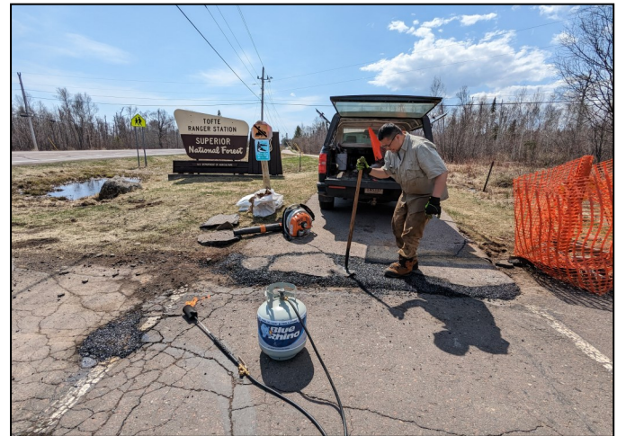
Oliver Liu repairs winter damage to the trail in Tofte this spring.
